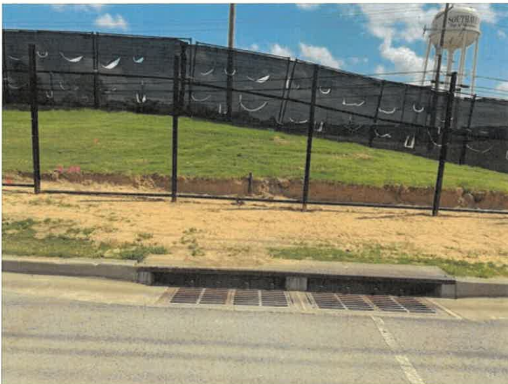
Photo 10-Another view of fence construction a little further east. Note ground excavation/leveling and lack of storm drain protection.
