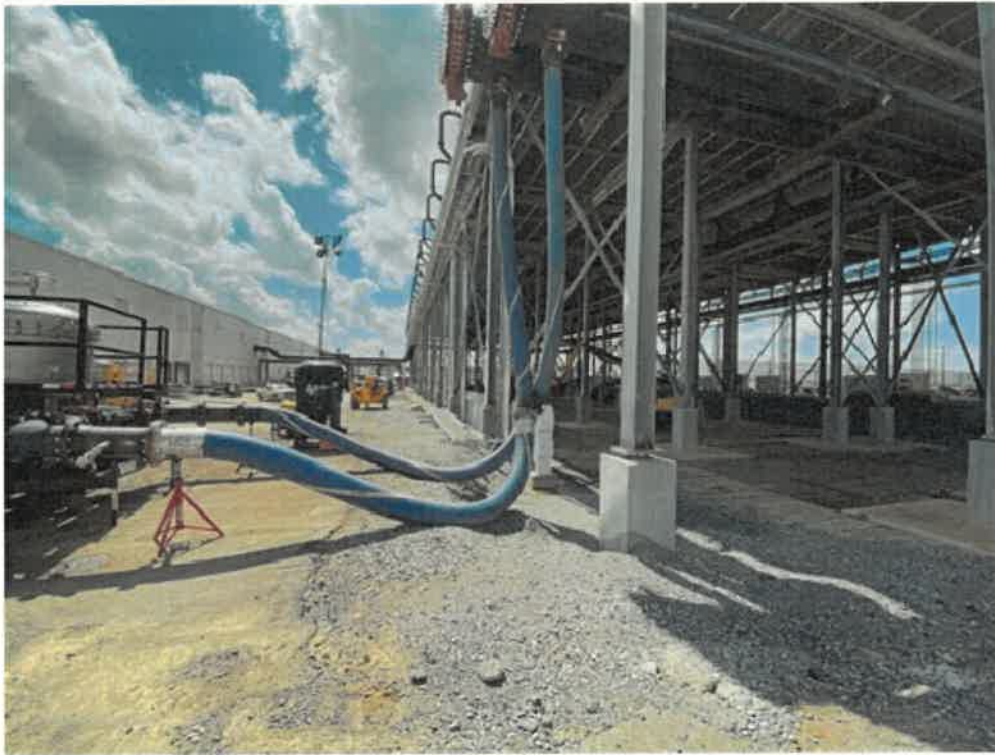
Photo 5-Looking west from same location as previous photo. Horizontal pipes in background lead to cooling tower structure.
