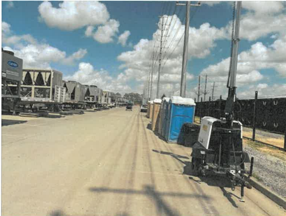
Photo 3-Mobile chiller/cooling tower units visible to left. These units surround the building on the west, east, and south sides.
