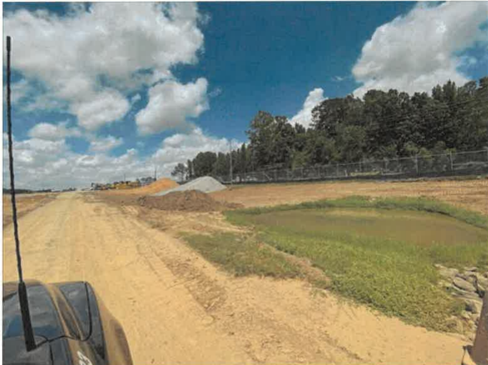
Photo 14-Material stockpiled along east fence with no controls.
