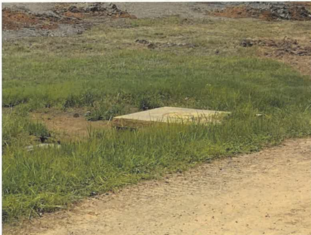
Photo 2-Unprotected storm drain; this was typical for other drains seen inside the fence.
