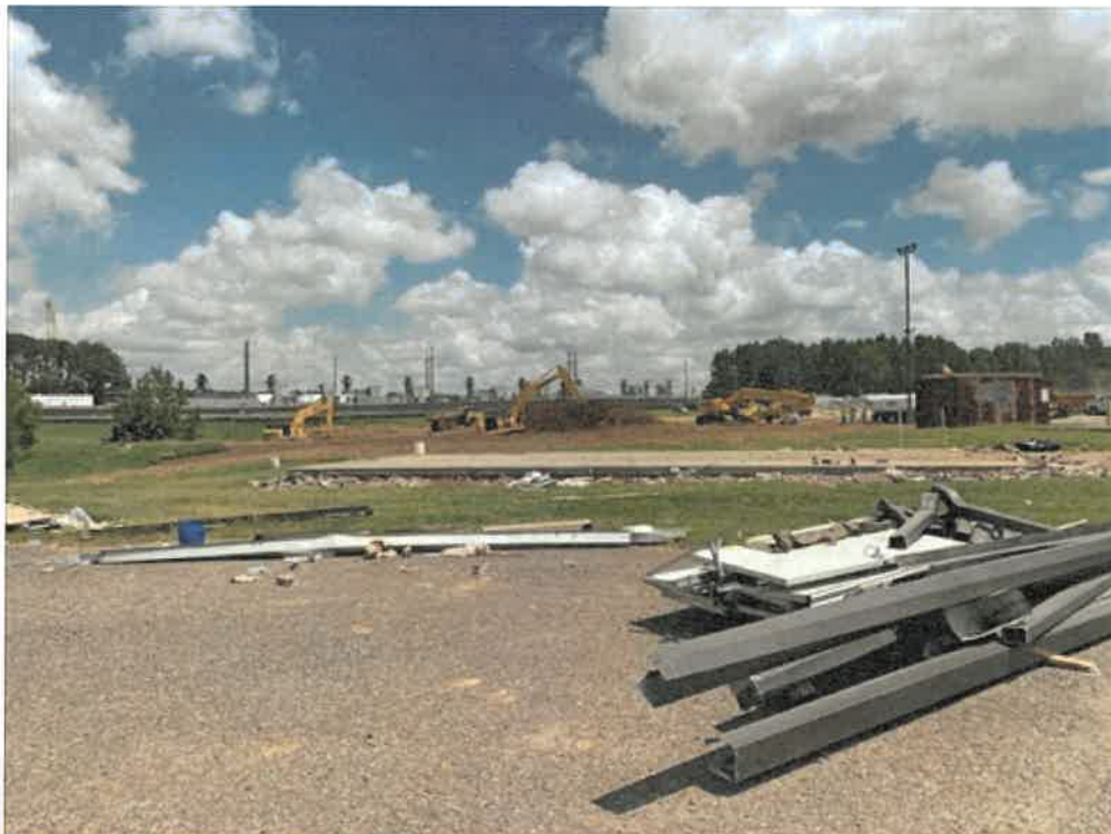
Photo 8-Remaining scrap and waste from recently-demolished buildings; looking east.
