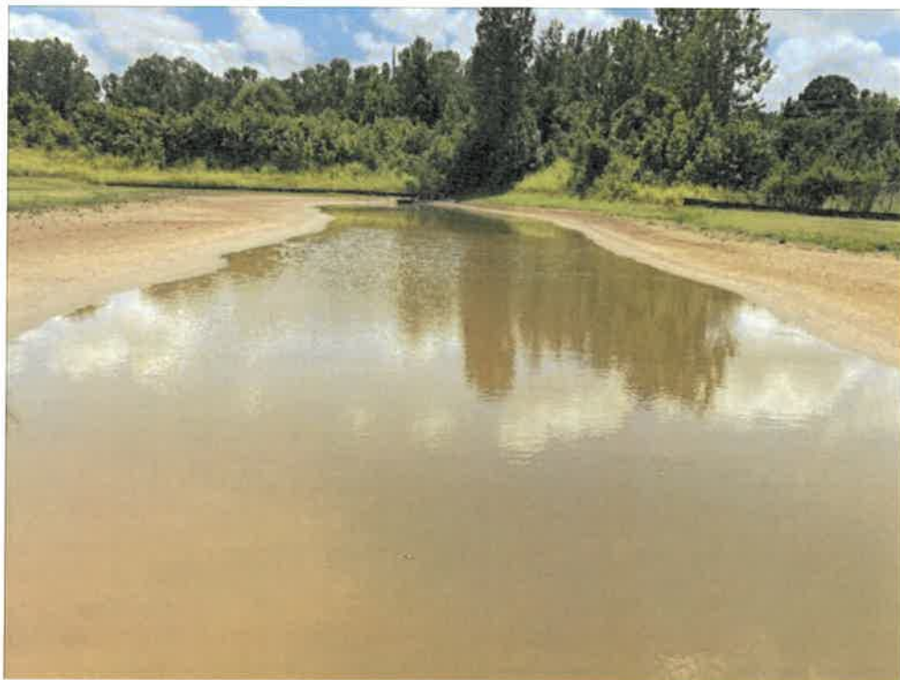
Photo 4-Looking south at last run of ditch flowing to Horn Lake Creek. Note lack of controls beyond perimeter silt fence.
